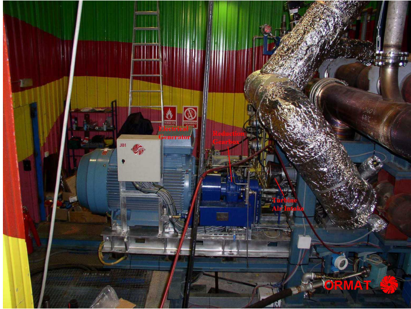
Fig. 2: PCU Commissioning at PSA
